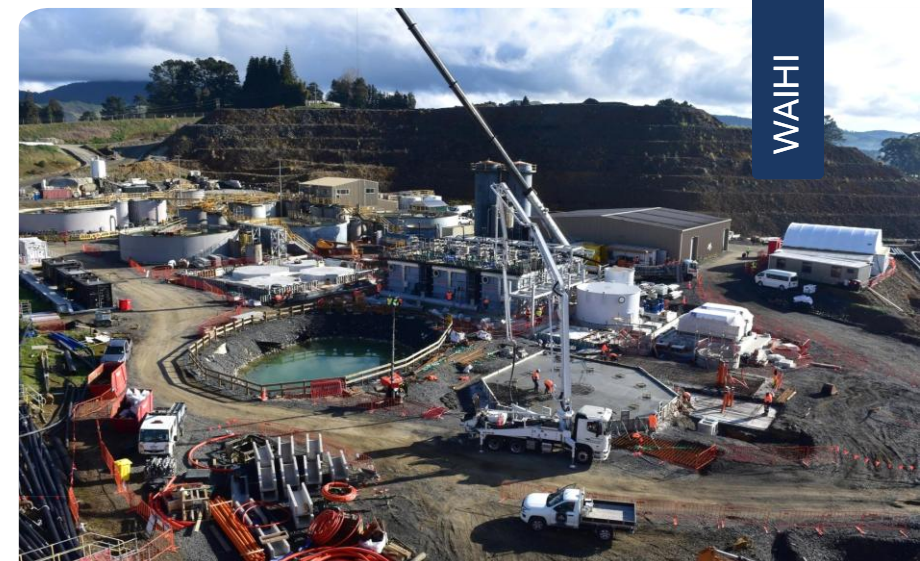
Water treatment plant – July 2026
